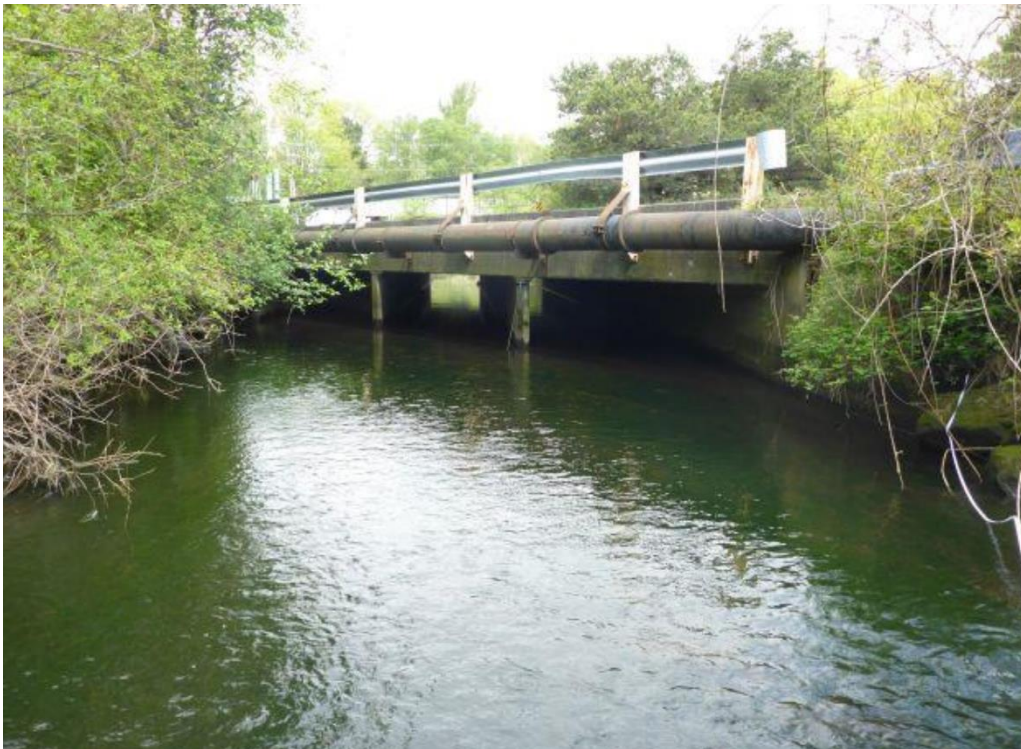
Figure 9. Roeder Avenue Culverts Looking Downstream to Culverts (top) and Looking Upstream to Culverts (bottom)
