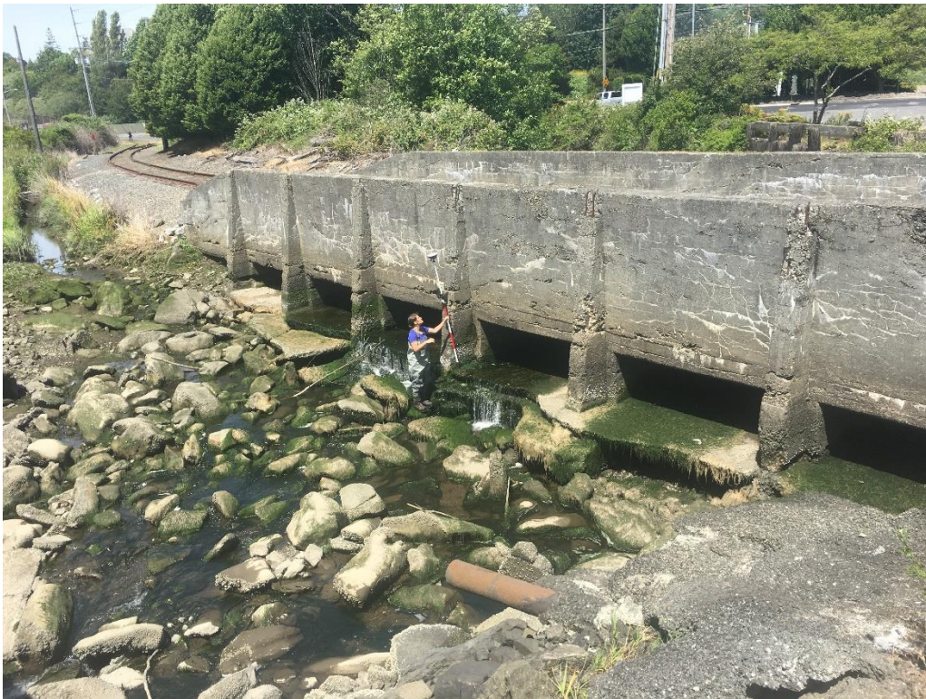
Figure 8. Railroad Spur Crossing Over Squalicum Creek Estuary at High Tide (top) and Low Tide (bottom)
