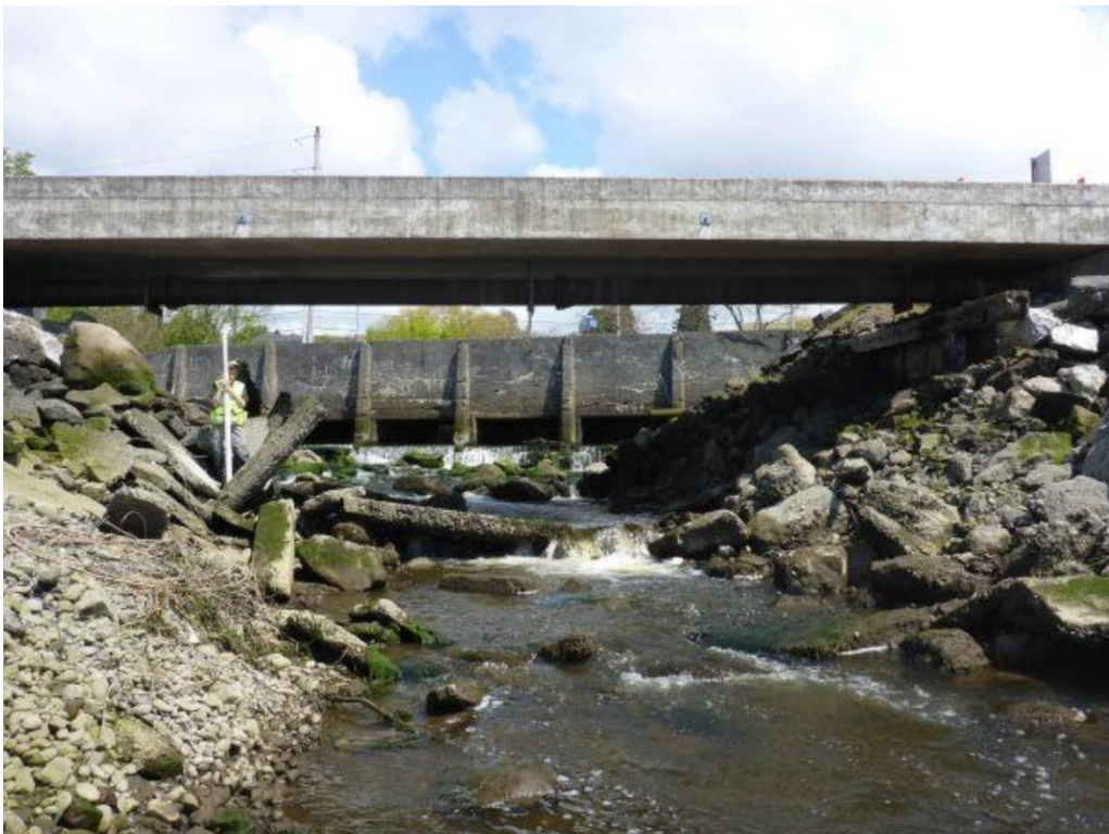
Figure 10. Port Bridge Looking Downstream at Bridge (top) and Looking Upstream at Bridge with Railroad Spur Crossing Culverts in Background (bottom)
