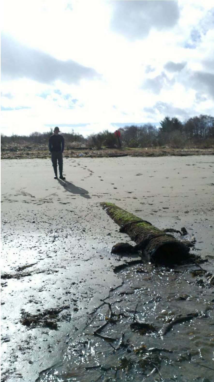
Figure 1. Example of culvert that backwaters by tide with outlet in the lower intertidal (Freeland Park Cr, stream # 36).
