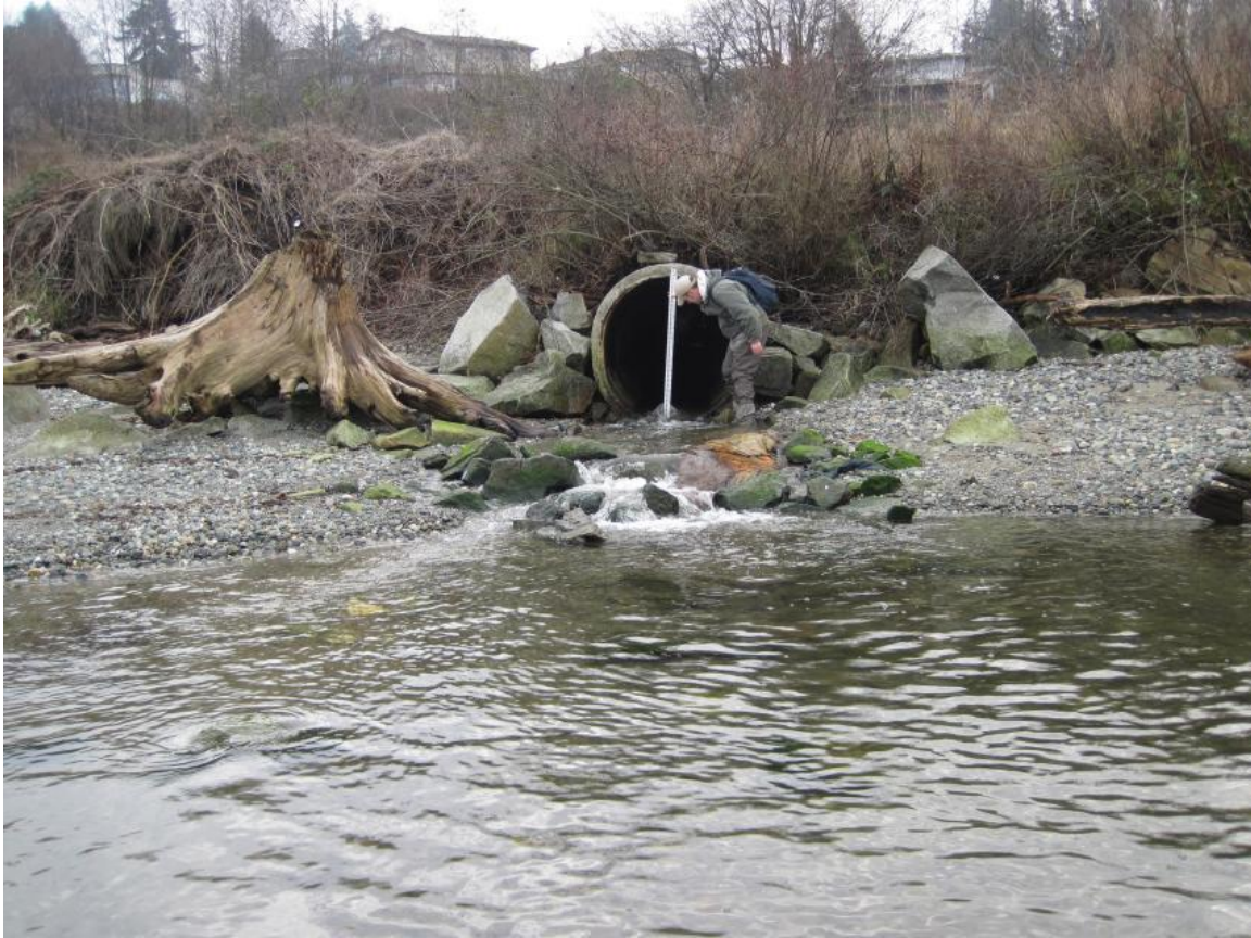
Figure 4. Example of culvert that backwaters by tide with outlet in the upper intertidal (Glenwood Creek, stream #46).
