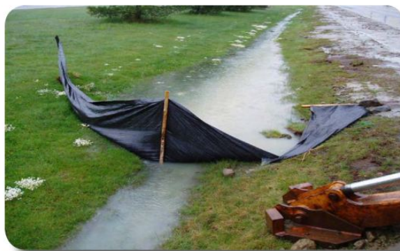
Poor erosion control can add sediment.
